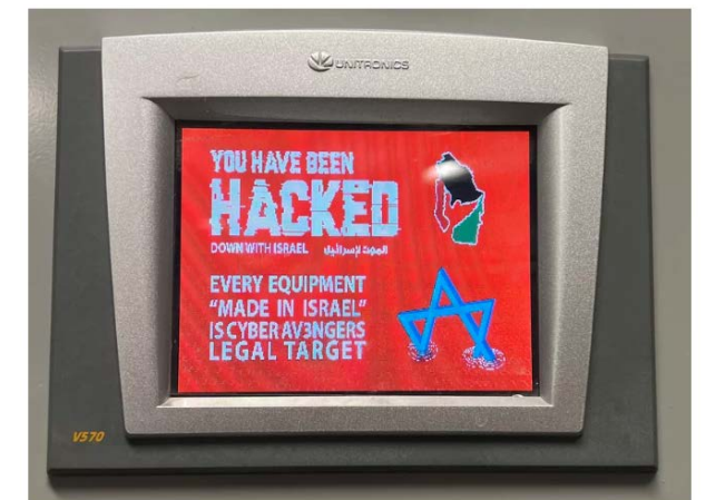
This photo provided by the Municipal Water Authority of Aliquippa shows the screen of a Unitronics device that was hacked in Aliquippa, Pennsylvania on November 25, 2023.
