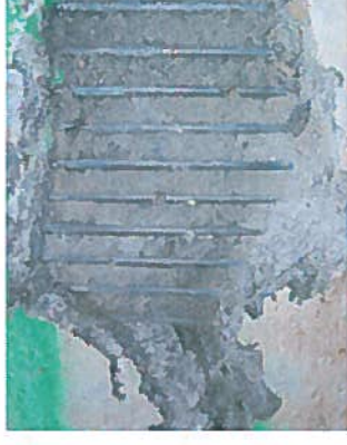
Broken wires – SW Transmission Main
