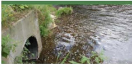
Combined Sewer Overflow
